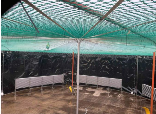
The interior of an anaerobic digester tank at the Beresford site is seen during construction. Manure is heated and sits in the 2-million gallon tanks for three weeks, letting off methane gas that's captured and refined for vehicle fuel. Submitted photo
