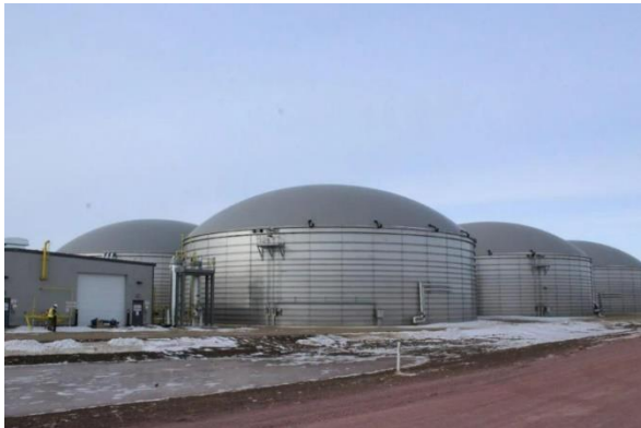
Four anaerobic digesters sit between two dairies north of Beresford, S.D. They use manure from 15,000 cows to make biogas for natural gas fleet vehicles in California. The farmer gets paid and the facility owners, DTE Vantage, make money off of renewable fuel credits. Tri-State Neighbor photo by Janelle Atyeo
