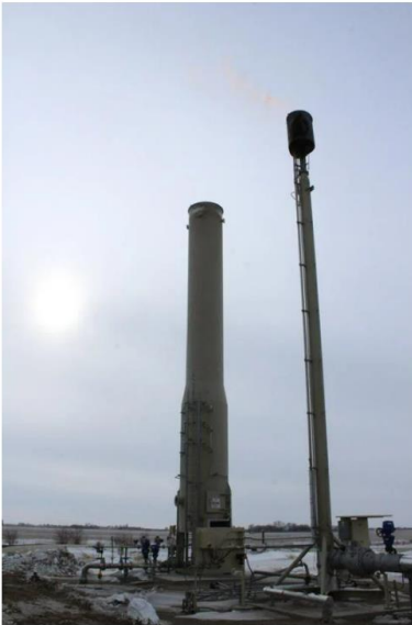
Flares burn off unwanted hydrogen sulfide and carbon dioxide gas after using methane from dairy manure to make renewable natural gas. Tri-State Neighbor photo by Janelle Atyeo
