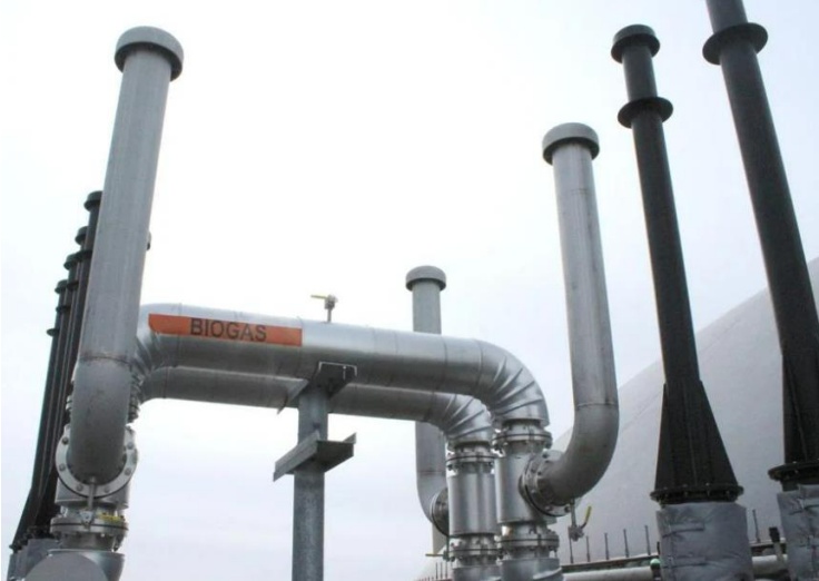
Pipes carry biogas from digesters near a dairy in Beresford, S.D. After a cleaning process, the renewable natural gas joins a pipeline that supplies transportation fuel to vehicles in California and other western states with renewable fuel targets. Tri-State Neighbor photo by Janelle Atyeo
